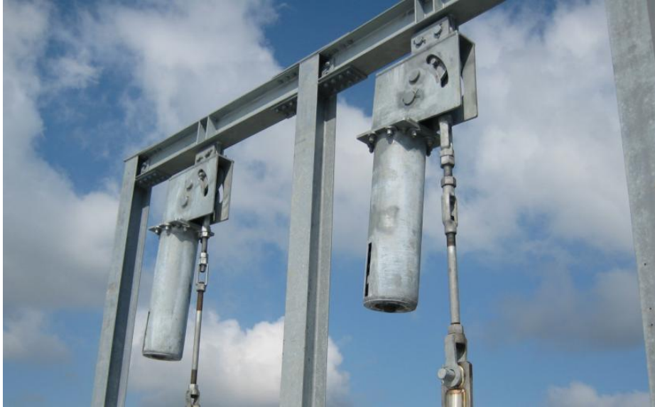
Figure 42: Spring hangers at the very top edge of an LNG tank – difficult to service but important to service
